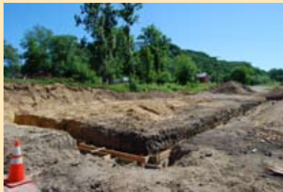
Gays Mills: The engineers are waiting for approval of the steel structure.
